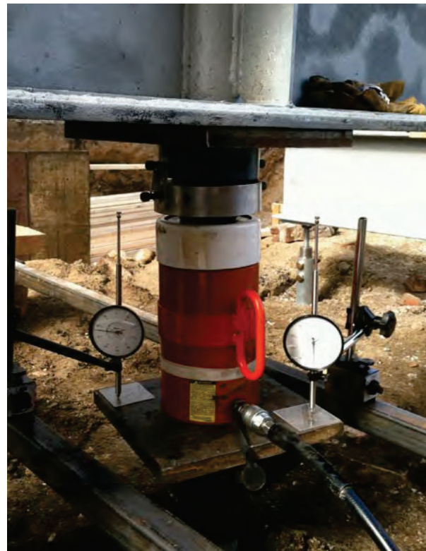
Figure 1.55 Close up of test pile, hydraulic cylinder, dial gauges and hemispherical bearing plate
