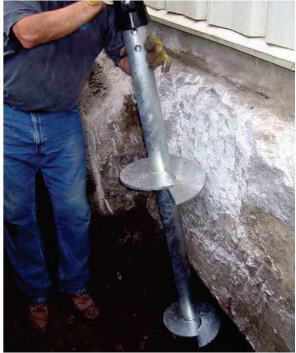
Figure 1.79 Alignment of lead
